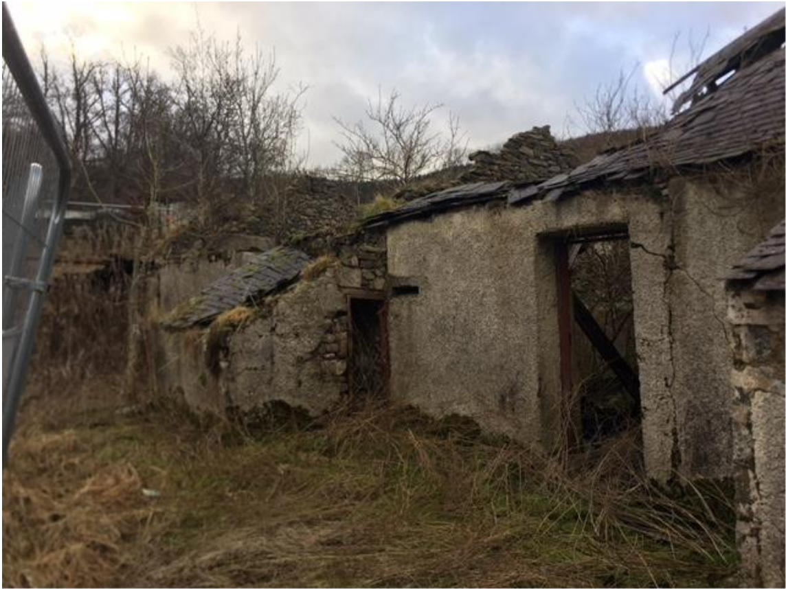
Figure 12: Image of the existing outbuildings attached to the Dwelling House falling into a state of disrepair
